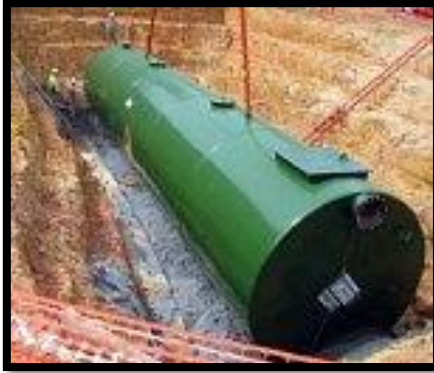
Figure 24. Underground Steel Tank
